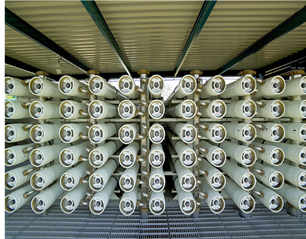
Reverse Osmosis Membranes at West Basin Municipal Water District, Brewer Desalination Facility. Desalination of local brackish groundwater helps reduce the Region’s dependence on imported water.
