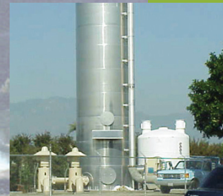
San Gabriel Valley Water Company's Plant No. 8 treatment facility in South El Monte.
